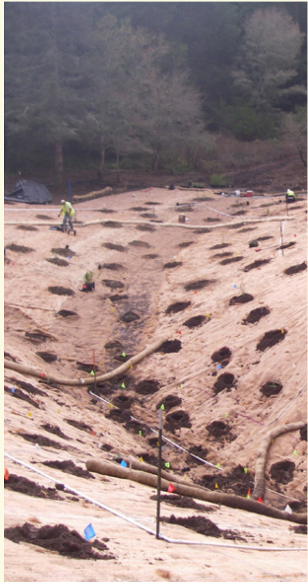
Blue Trail Gully just after completion of the gully repair project. Since then, the site has revegetated and the impacts of the gully are no longer visible. Credit: Balance Hydrologics, Inc.
